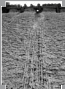
Fig. 13 : Decay caused by leaky eaves (C. Ziegert).
